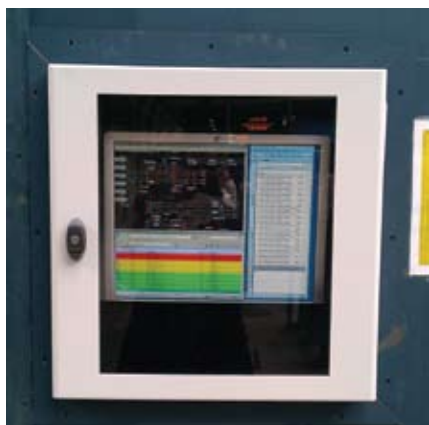
Enclosure Installed in Temporary Hoarding at Kings Cross P 5&6
